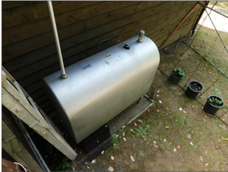
Photo 3 – Heating oil AST adjacent to the west wall of Site Building A.
